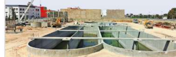
Figure 1: Aeration basin under construction at the Nouaceur wastewater treatment plant in Nouaceur, Morocco
