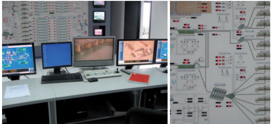
Figure 24: A water utility control room (Festo Didactic)
