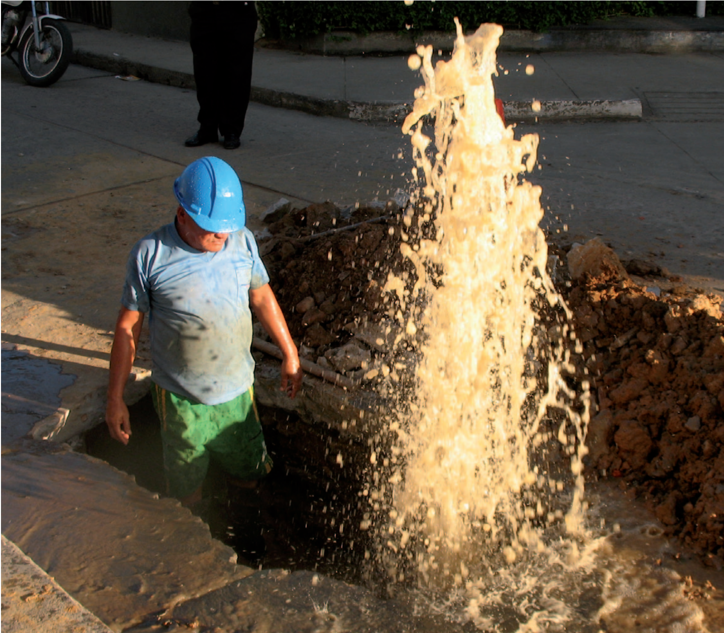
Figure 23: Water leak in Lima (Hermann Sewerin GmbH)
